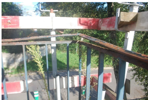
Figuur 28: Loskomen verf/coating balustrade
